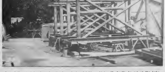
One of the steel bridges for the Superstrata pipeline which will shortly be set at the Lake Tashor dock No. 1 is shown above at the Battifield. One of the dolphins was made at the Builder Shop, and another at the Welding Shop. The other two will form the foundation of Lake Tashor dock No. 1.
